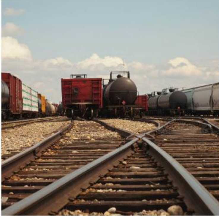
Railroad ties act as beams that support very large transverse shear loadings. As a result, if they are made of wood they will tend to split at their ends, where the shear loads are the largest.
